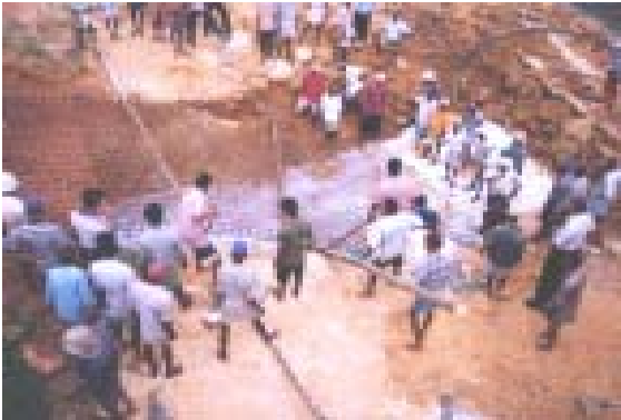
Top Women and children working on the Kiriwalagama crossway bridge >> Community and skilled tradesmen working together to lay the foundations for Kiriwalagama's crossway bridge
