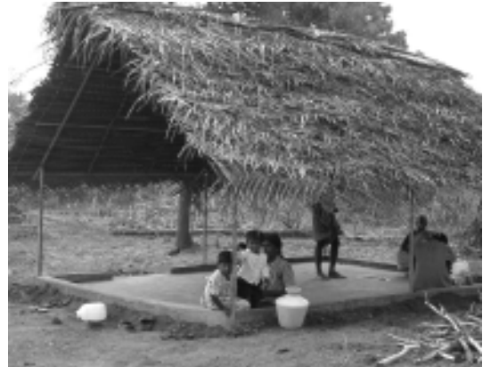
Temporary shelter being constructed for a returning family in Vavuniya North with a GAA/BMZ & Sewalanka partnership
